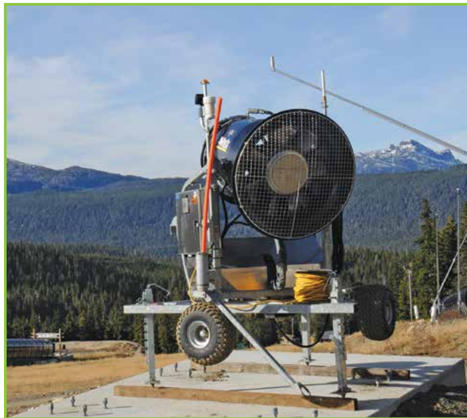
Operations crews have spent the past few months burying pipes and installing snow guns for some serious snowmaking at Mount Washington Alpine Resort this winter. Susan Quinn Photo
