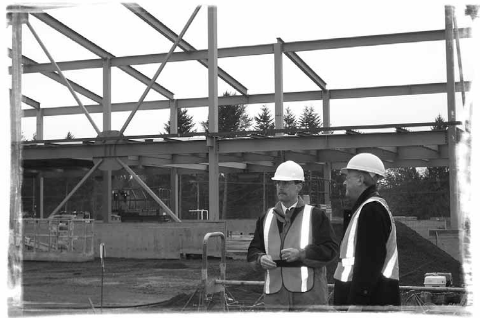
Project Co-ordinator Blair Pettis and MLA Stan Hagen review the construction progress of the new Comox Airport Terminal.
